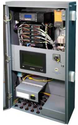
415/220V LV RTU
