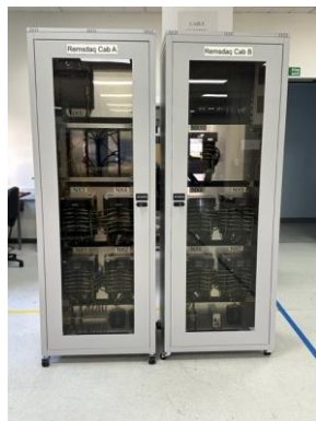
Substation Automation System
