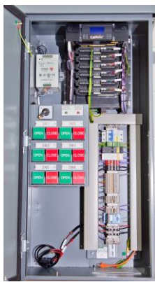
11kV RMU/OH 1-6 Switches
