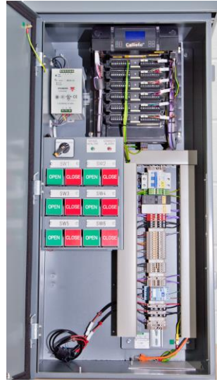
11kV RMU/OH (1-6 Switches)
